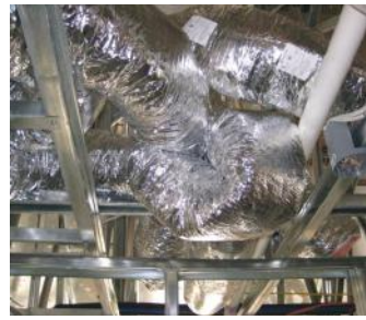
Ducts are crammed into cavity, kinked and sharply bent.
