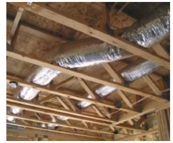
Ducts are run straight and supported properly.
